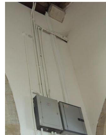
The location of electrical equipment and wiring runs all needs careful consideration with professional advice
