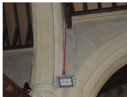
The choice of cable, colour and wiring runs may have a dramatic effect on the appearance of a church
