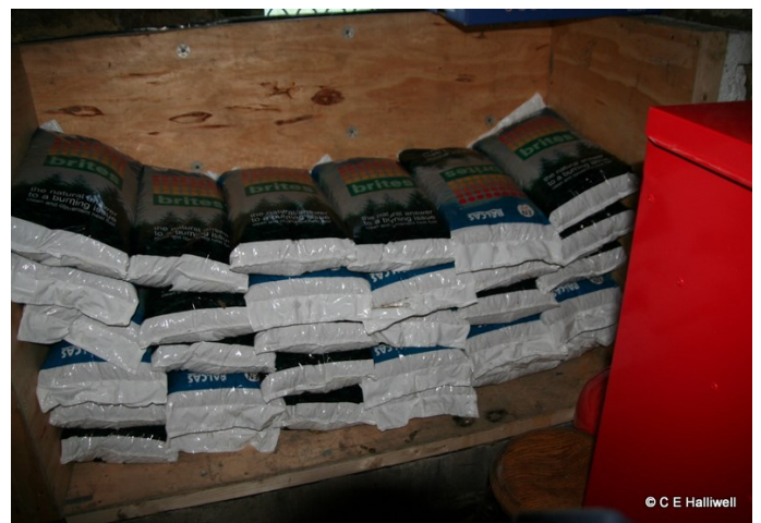
Above: Tatham Fells, Good Shepherd Church: biomass boiler, hopper, and wood pellets
