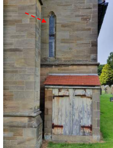
b) Weathered doors and corroded hinges. Broken secondary glazing.
