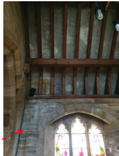
b) Salt staining and defective ceiling panels.
