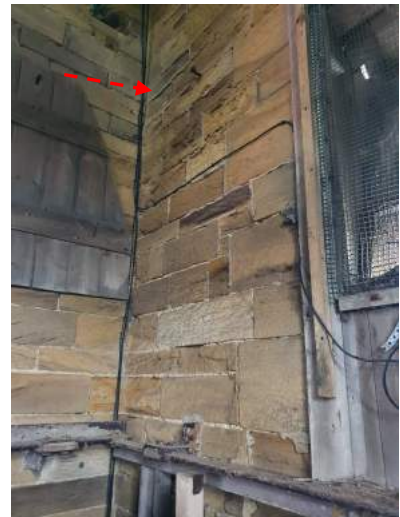
b) Surface erosion to masonry
