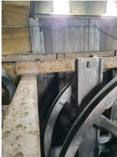
a) Bell frame corrosion
