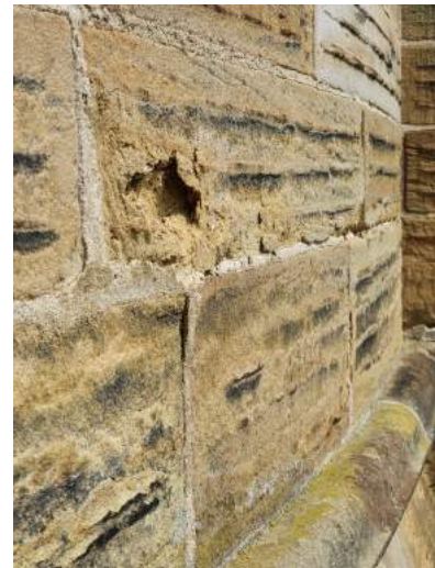
b) The use of inappropriate mortar for previous repairs is probably contributing to the masonry erosion starting to develop.
