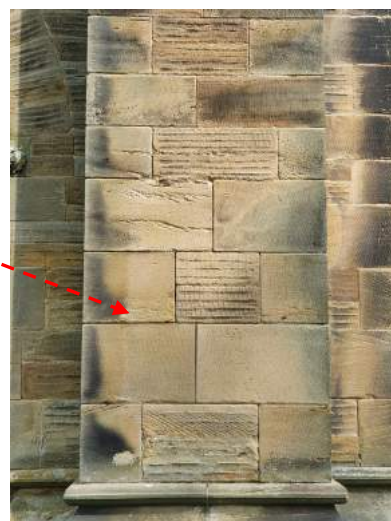
b) Mortar is washed out of joints and ought to be repointed.
