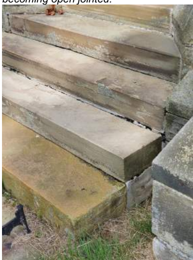
a) Steps would benefit from repointing.
