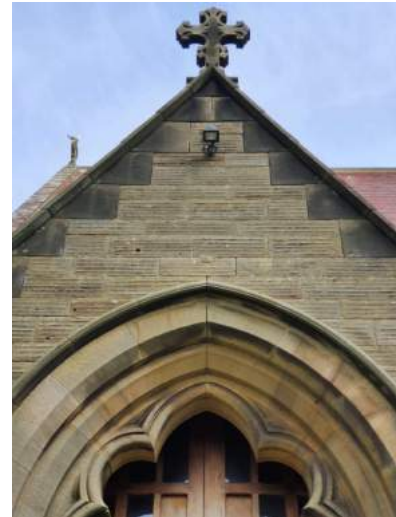
b) Mild erosion starting to occur in the perp joint below the finial cross and apex of the arch doorway.
