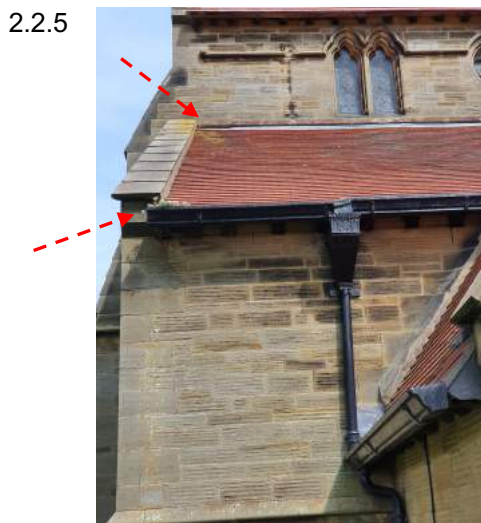
a) Distorted lead and vegetation in gutter
