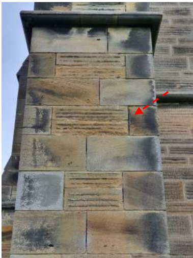
a) Prep and bed joints to buttresses have lost mortar.
