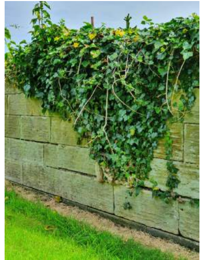
b) East boundary – ivy has grown through the wall and is damaging its construction. The vegetation needs to be cut back, controlled and the wall repaired.
