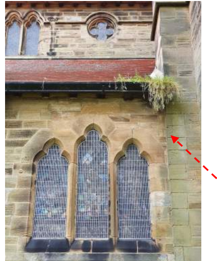
b) Clear gutter to prevent further spillage and staining.
