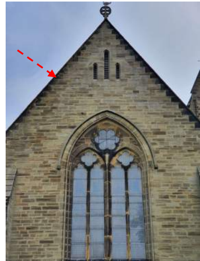
b) Mortar loss to coping blocks
