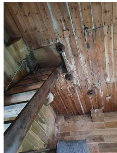
b) Hatch to belfry is awkward to open. Note stained ceiling boards.
