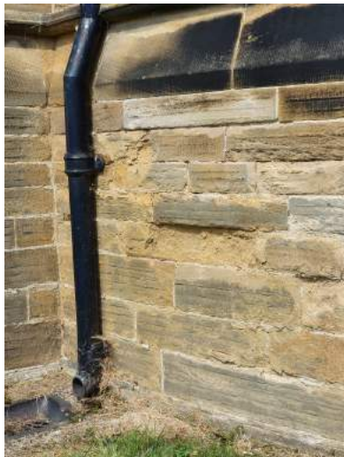
a) Repointing and mortar repair required,
