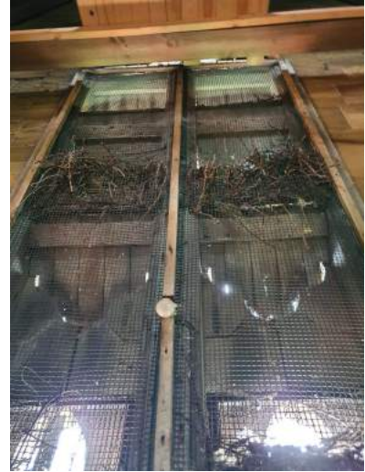
b) Nest established between louvres and mesh.
