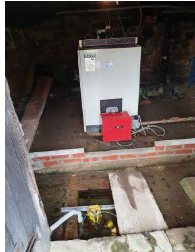
b) New pump and flood wall
