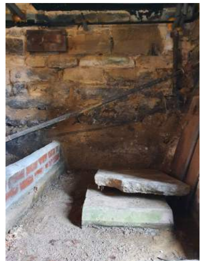
b) Walls are floor are damp for much of the year.
