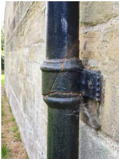
a) Fractured bracket/ pipework
