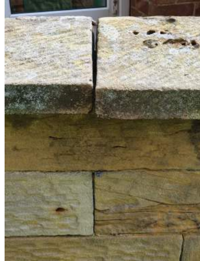
b) Open jointed/ displaced coping to east boundary ought to be repointed
