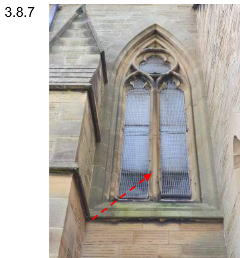
a) Masonry repair needed
