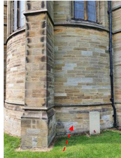
b) Salting due to rising damp is causing erosion in the plinth
