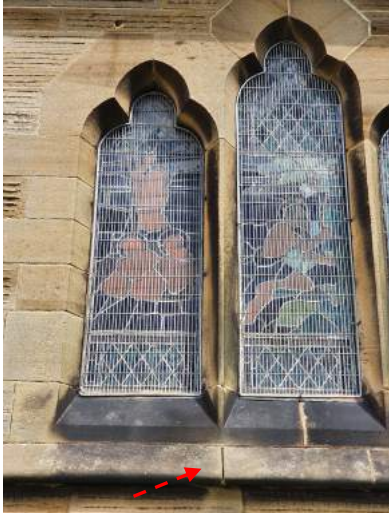
a) Open joints to need to be repointed
