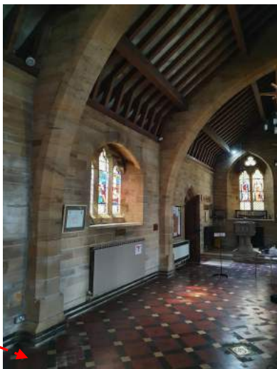
a) Mild salt deposit on floor tiles
