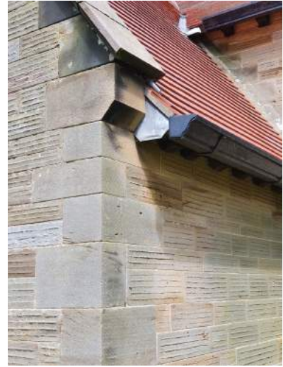
b) Mild erosion to bed joints between quoin stones
