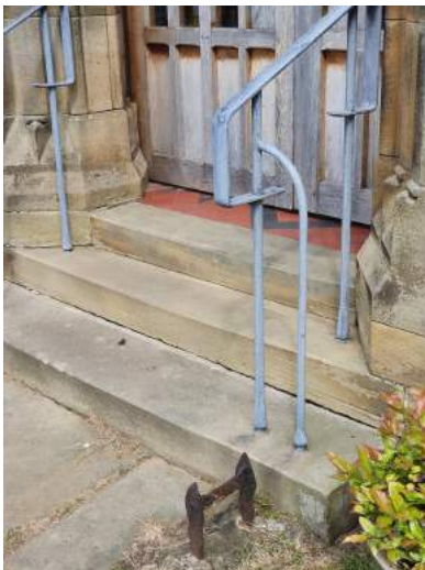
a) Bottom steps slightly open jointed.
