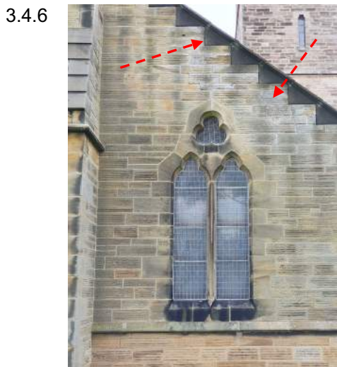
a) Open jointed coping blocks and salt staining.
