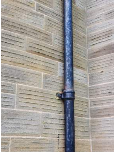
a) Ironwork to be brushed down and redecorated
