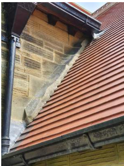
a) Mortar haunching thought to cover lead flashing below.
