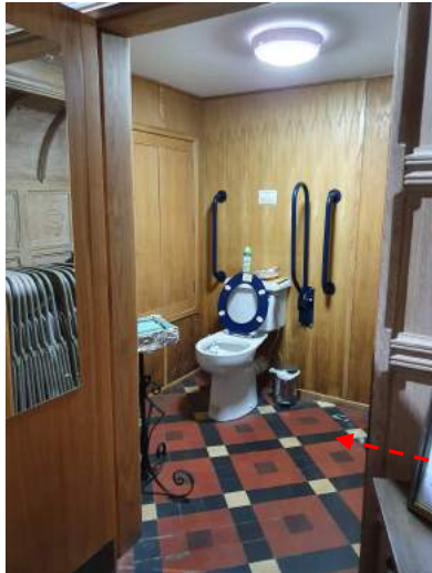
a) WC – Salt deposits of tiled floor
