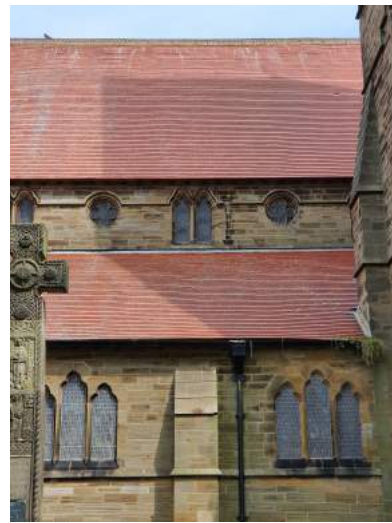
b) Gutter droops at east end
