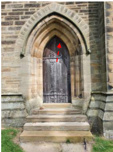
a) Voussoirs are losing mortar and becoming open jointed.
