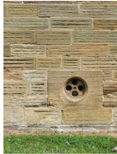
b) Low level masonry is showing some salt deposits and minor erosion due to rising damp
