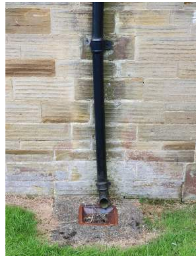
b) Downpipe is misaligned and the adjacent masonry is stained. Refurbish all downpipes and gutters checking for leaks.
