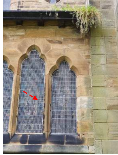
b) Window guard fixings are damaging the mullions. Are window guards necessary?
