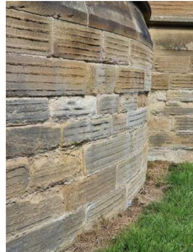
b) Masonry and mortar erosion
