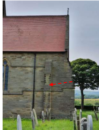
b) Buttress requires repointing
