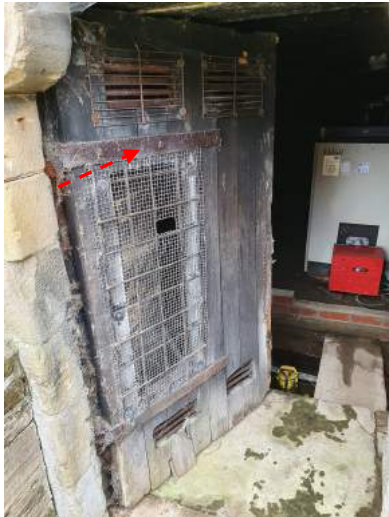
a) The basement door is rather dilapidated but functional.
