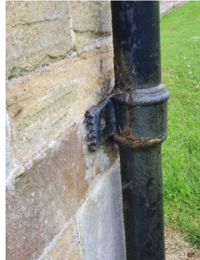
b) Fractured cast iron
