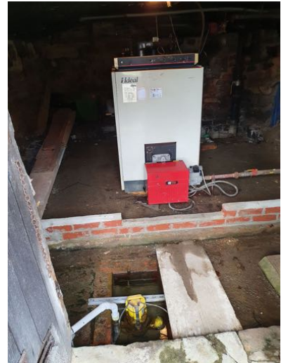
b) New pump and flood wall
