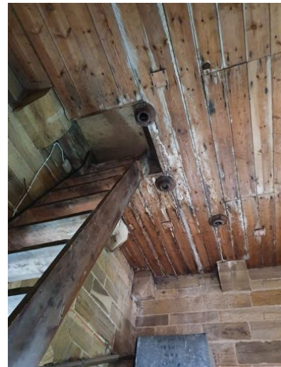
b) Hatch to belfry is awkward to open. Note stained ceiling boards.
