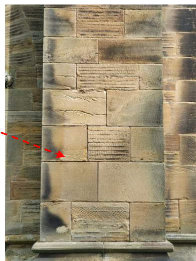
b) Mortar is washed out of joints and ought to be repointed.
