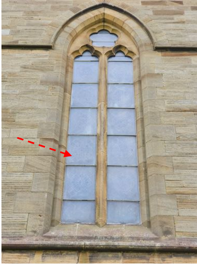
a) Exterior secondary glazing is cracked
