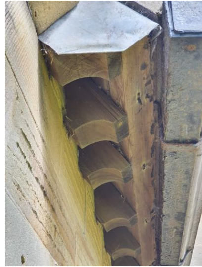
b) Exposed rafter ends in fair condition.
