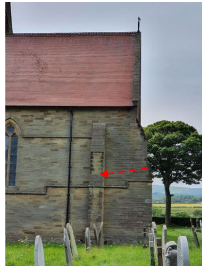
b) Buttress requires repointing
