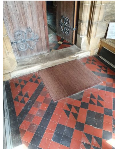
b) Open perpendicular joints and surface erosion caused by rising damp.
