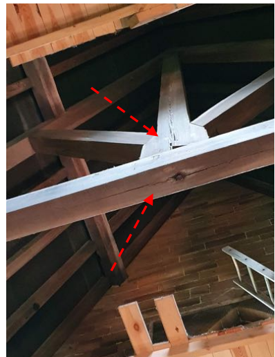
b) Split at the base of the centre post and to the underside of the bottom chord.
