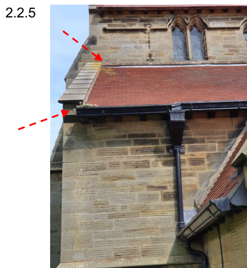
a) Distorted lead and vegetation in gutter
