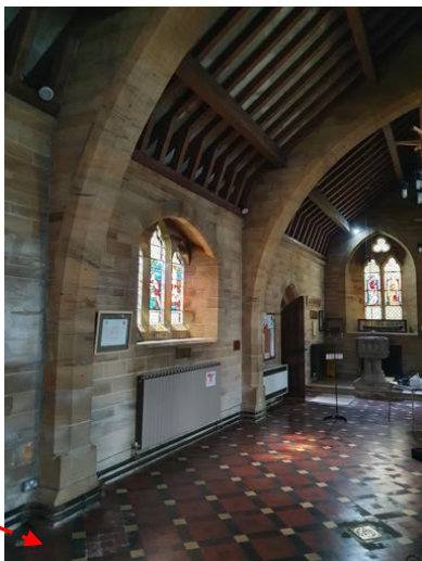
a) Mild salt deposit on floor tiles
