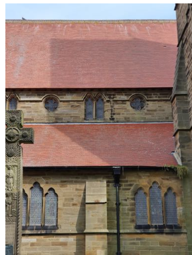
b) Gutter droops at east end
