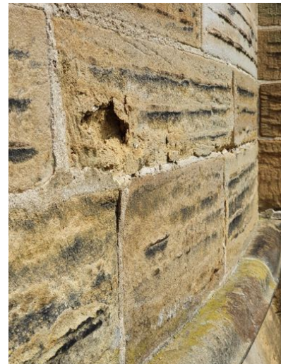
b) The use of inappropriate mortar for previous repairs is probably contributing to the masonry erosion starting to develop.
