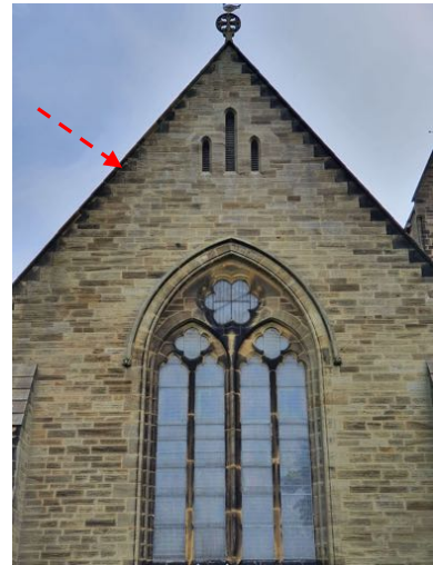
b) Mortar loss to coping blocks
