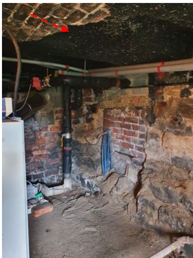
a) Surface coating to brick vault is breaking down
