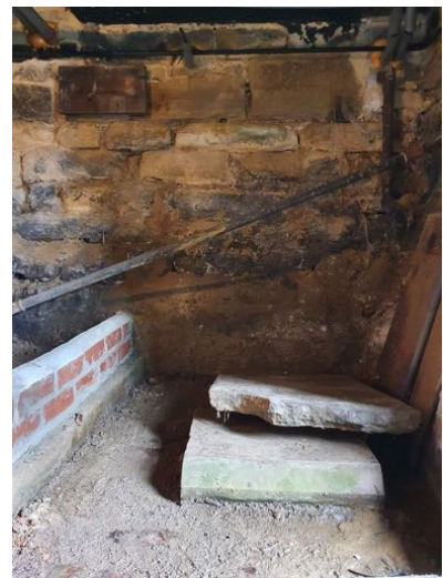
b) Walls and floor are damp for much of the year.
