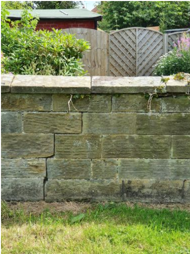
a) Open joints form stepped crack in east boundary wall that ought to be repointed
