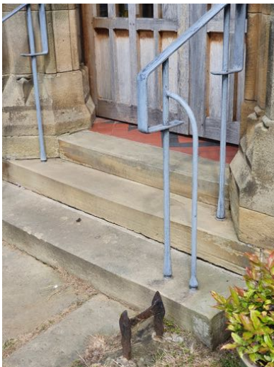
a) Bottom steps slightly open jointed.
