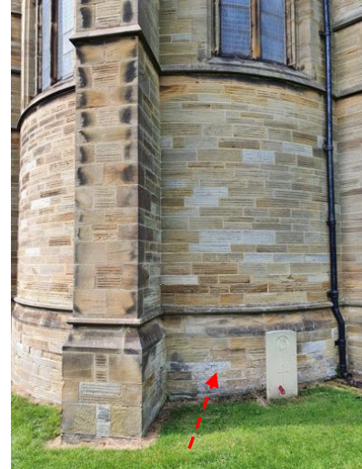
b) Salting due to rising damp is causing erosion in the plinth
