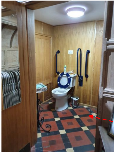
a) WC – Salt deposits of tiled floor
