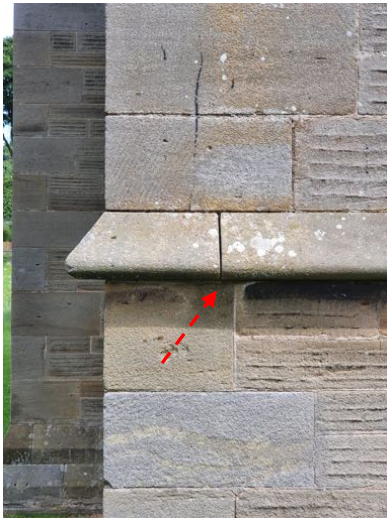
a) Mortar has washed from joints on exposed corners.
