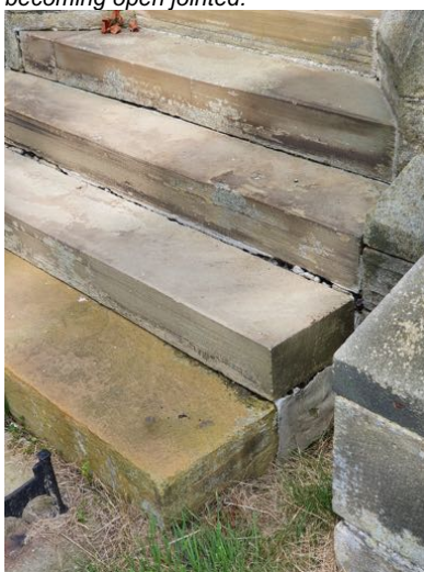
a) Steps would benefit from repointing.
