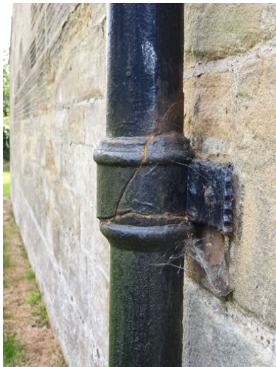
a) Fractured bracket/ pipework
