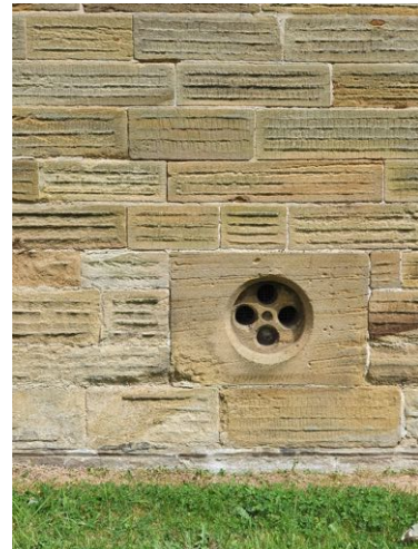
b) Low level masonry is showing some salt deposits and minor erosion due to rising damp
