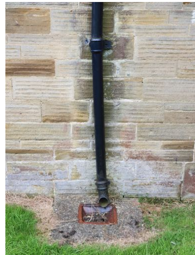
b) Downpipe is misaligned and the adjacent masonry is stained. Refurbish all downpipes and gutters checking for leaks.
