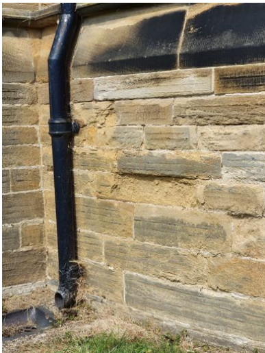
a) Repointing and mortar repair required,
