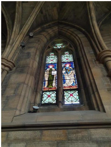
a) North apse window central mullion has been repaired but shows signs of continuing erosion that reflects the location of external masonry defects
