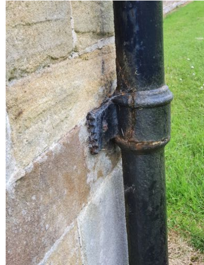
b) Fractured cast iron
