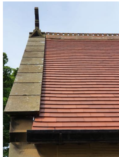
b) Finial cross appears to lean forward slightly.
